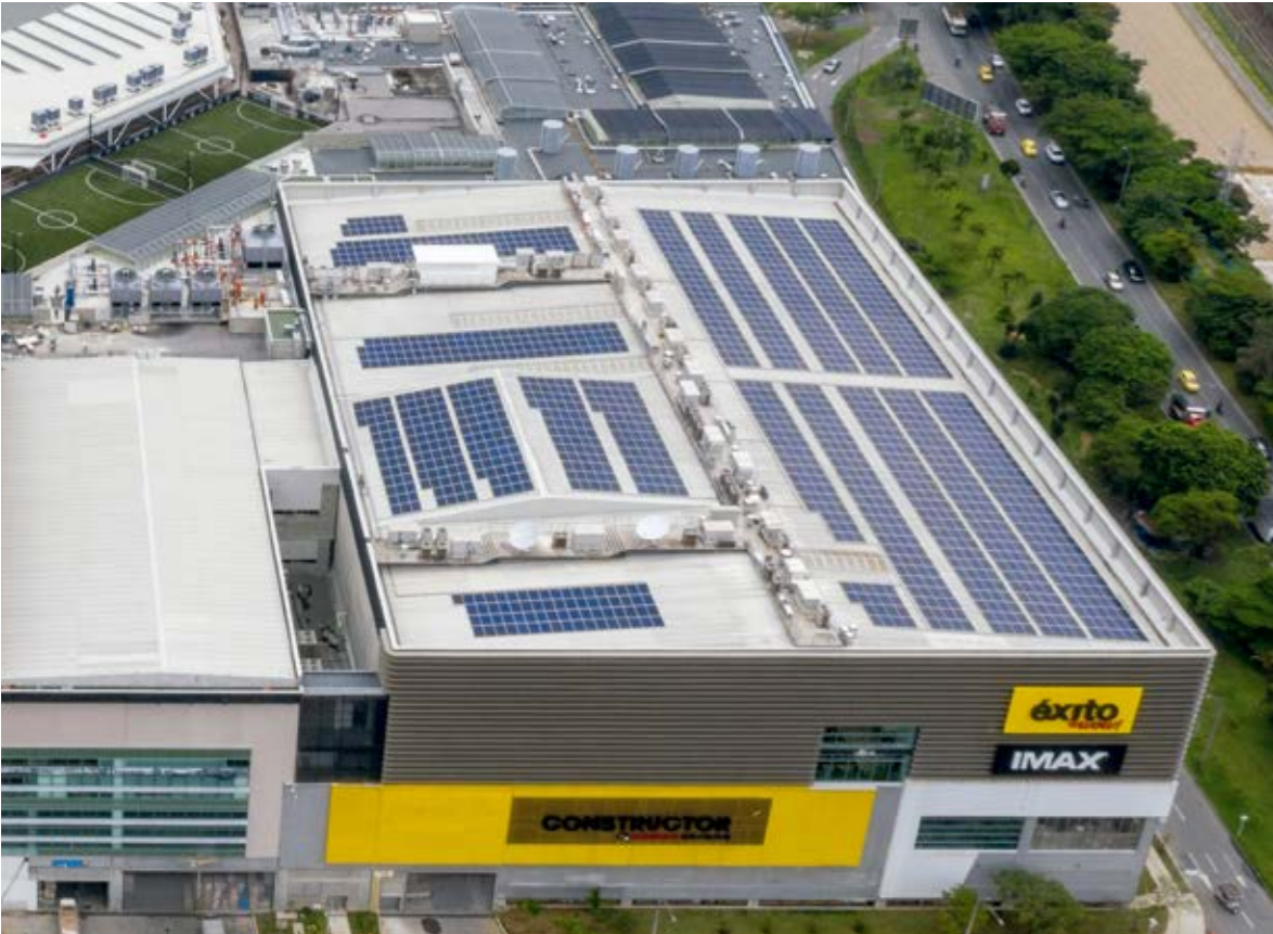
Viva Envigado has the fifth photovoltaic plant in the Company. It generates more than 451 kw/h with 2,700 m 2 of solar panels and supplies up to 20% of consumption in the common areas of the commercial complex during maximum sun radiation hours
